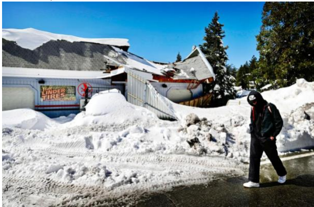
A man walks by Linder Tires, where the roof collapsed due to the weight of the snow in Crestline on Friday, March 3, 2023. (File photo by Watchara Phomicinda, The Press-Enterprise/SCNG)
