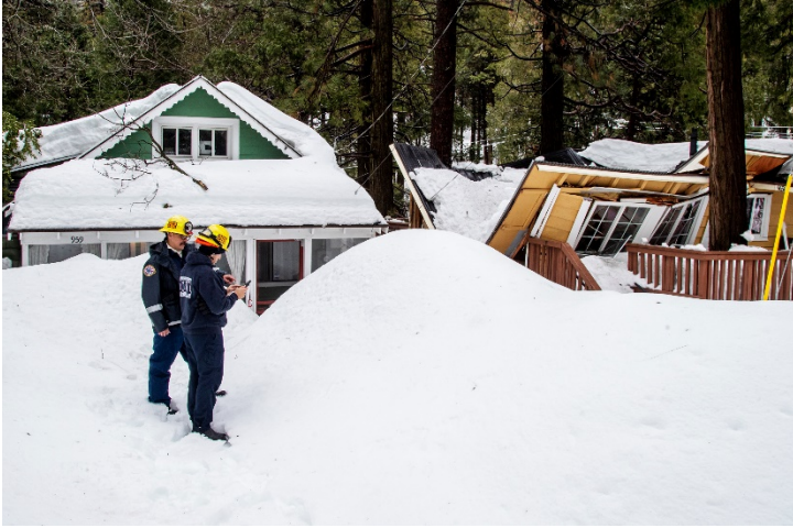
Fire crews document the damage to a house with a collapsed roof in Crestline, Calif., on Monday.
