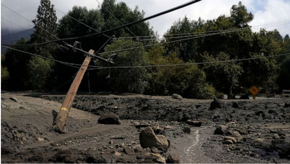
Electric poles are seen half-fallen in the aftermath of a mudslide, Sept. 13, 2022, in Oak Glen, Calif.
