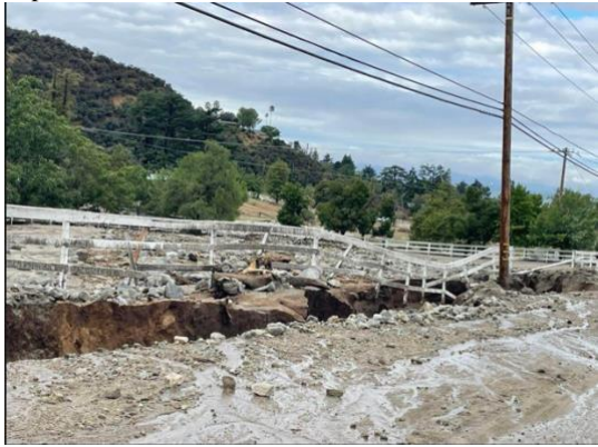
Oak Glen Road has major damage from the storm last week
